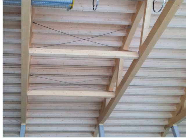
The stabilizing construction absorbs the forces of the sports equipment
