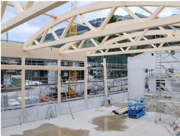
More supporting structure height due to the slightly upward curved bottom chord of the trusses
