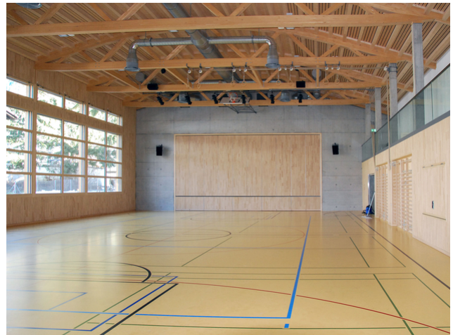
Sufficient space for the ventilation pipes thanks to the truss construction
