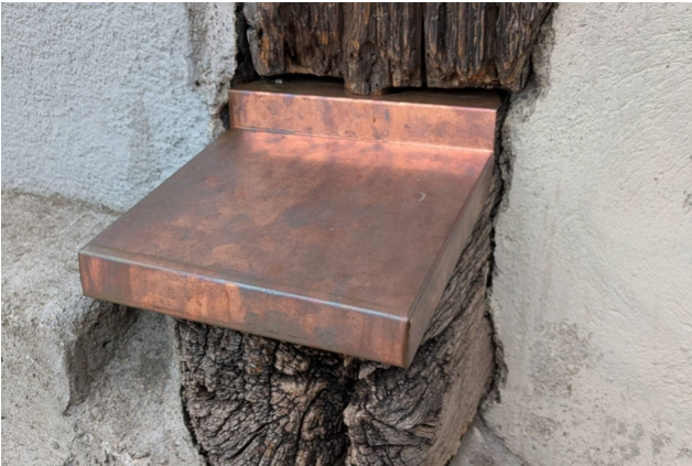
Constructive wood protection helps to protect the half-timbered structure from moisture penetration.
