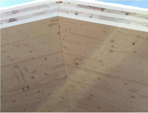
Snapshot of the construction work: Cutting together the roof panels in the ridge area
